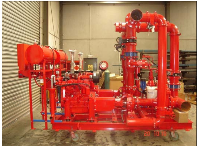
Packaged fire pump set built by Rob Laine for Leemark Fire Protection. (Pump duty 5,500 l/m @ 500 kPa, Southern Cross ISO125-250, Cummins 4BT 75 kW @ 2600 rpm).
